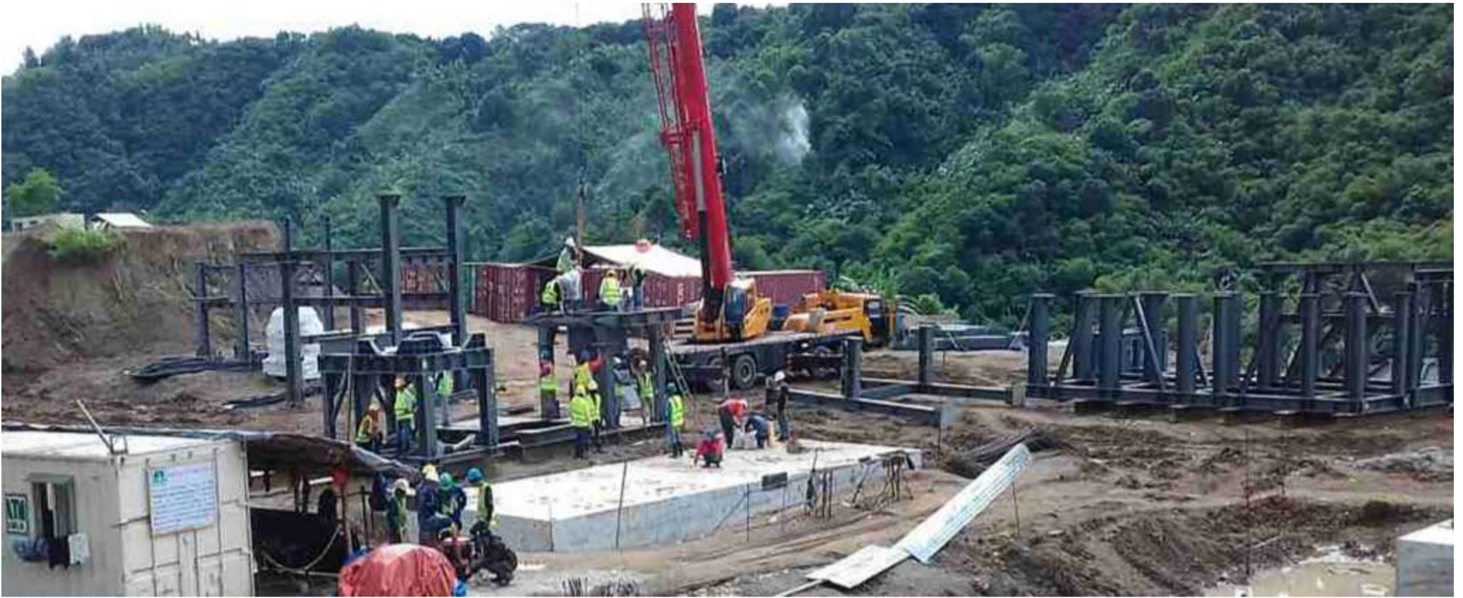
6-HECTARE ATN DEVELOPMENT AS OF OCTOBER 16, 2017 : (A) 2.5-HECTARE CRUSHER PLANT FOR 3.5 MILLION TONS OF PROCESSED ROCKS PER YEAR; (B) 2-HECTARE BOULDERS RAW MATERIALS STOCKPILE AREA; (C) 5,000 SQM SEMI-PROCESSED ROCK STOCKPILE UNDERGROUND CHAMBER; (D) SILT TRAPS AND SETTLING PONDS OF 1-HECTARE IN MONTALBAN, RIZAL
