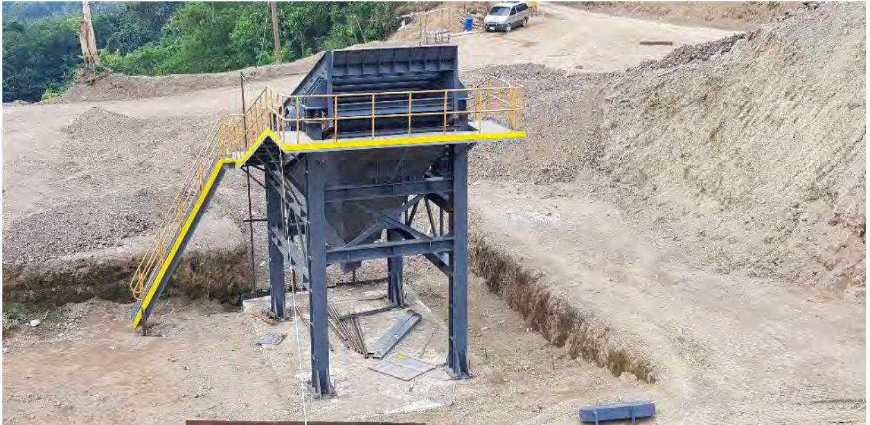
The product screening station (the 2 nd unit), now with toe board installed with “safety standard yellow color”
