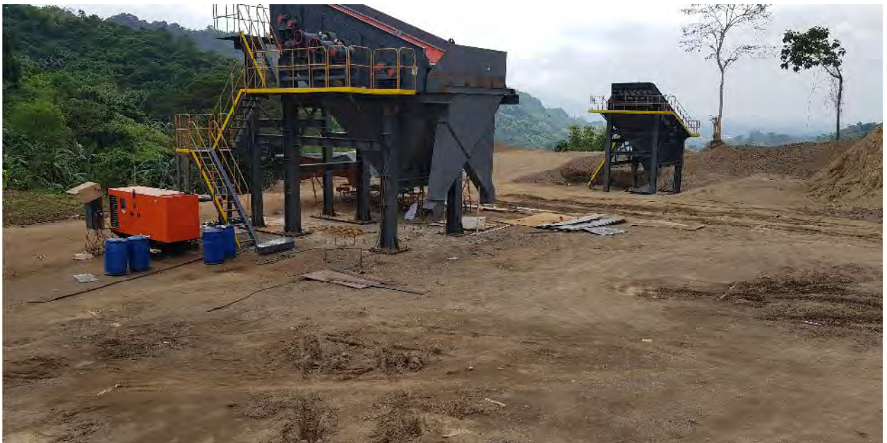
As shown, the screening stations were both have the toe boards installed (cut from your supplied steel plates, welded to these structures), applied with primary paint & now with “standard yellow final paints”.
